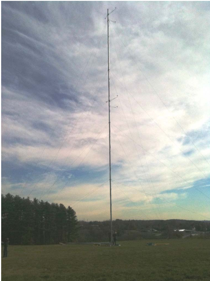
Figure 7: Photograph of the installed meteorological tower.
