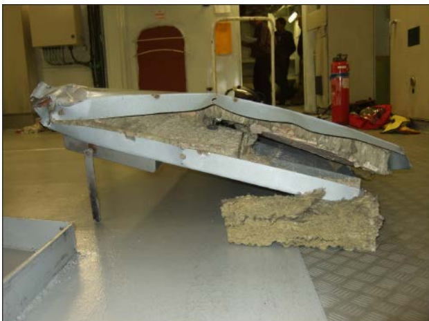
Fig. 18: Steel Door from Harmonic Filter Capacitor bank on Queen Mary II REF SB4-10
