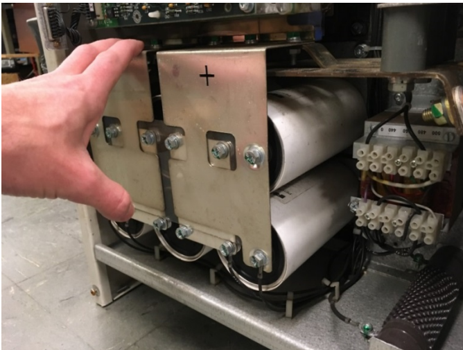
Fig. 15: DC Link Capacitors on 100 hp Inverter
