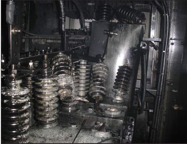
Fig. 17: Capacitor Explosion on Queen Mary II REF SB4-10
