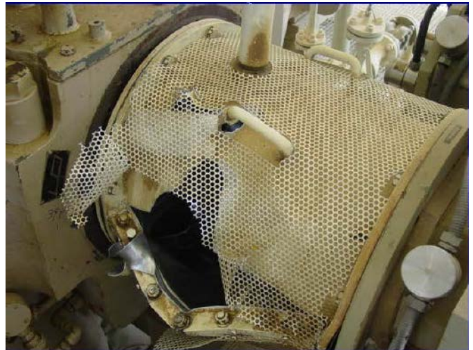
Fig. 19: VFD-induced Coupling Failure on 18000 hp LPG Compressor [15]
