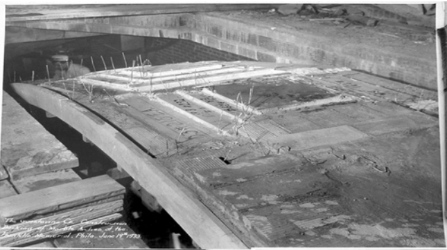
Figure 11. Installation of coffers in dome structure at the Benjamin Franklin Memorial, Philadelphia (1933) (Avery Library, Columbia University).
