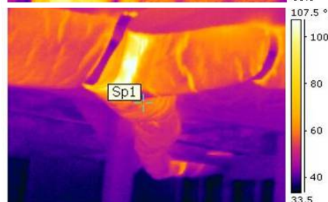
Infrared images of common home energy problems in a Berkeley home, each of which can be addressed through the RECO. Top: Heat loss under an exterior door. Middle: poorly insulated attic. Bottom: leaky forced air HVAC ducts.
