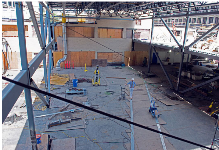
Building 31's new high-bay space will be home to the Center for Autonomous Systems, a place where AeroAstro researchers can conduct research involving flying robotic aerial systems. (William Litant/MIT photograph)
